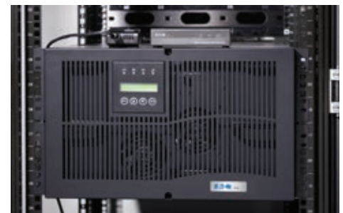
Environmental Monitoring Probe and Environmental Rack Monitor mounted on top of Eaton UPS
