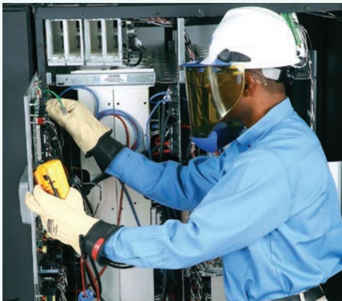
Proper preventive maintenance reduces the risk of UPS failure through thorough inspection, cleaning, testing and calibrating various electronic and mechanical components.
