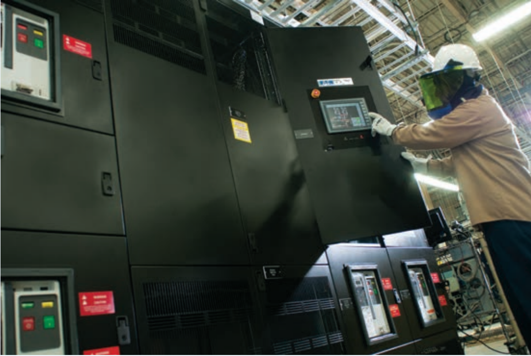
Eaton's Witness Test Centers allow you to see your large multi-module system tested before it's deployed.
