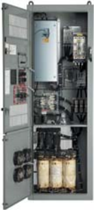
Enclosed 18-Pulse Drive
